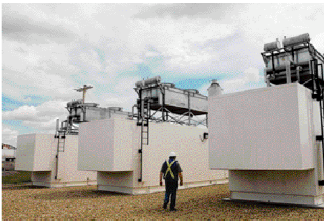
Electricity Generation from Landfill Gas
